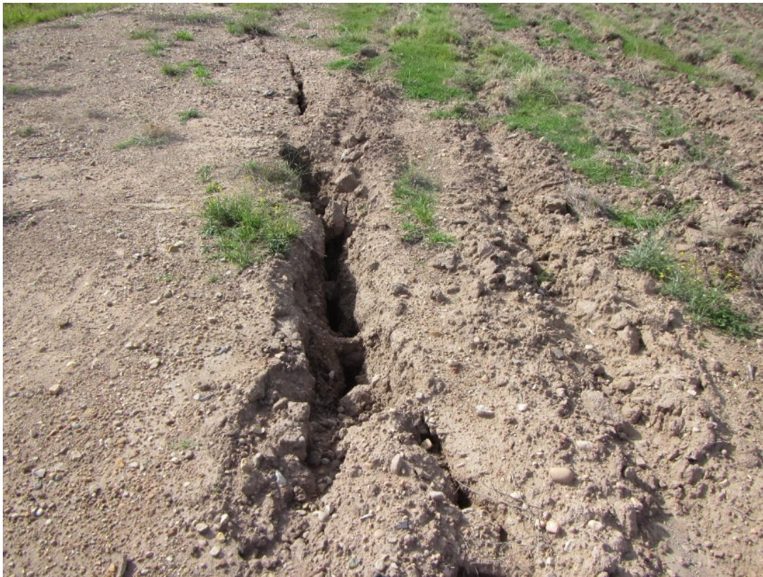
Figure 3-4. Cracking at surface over LW13/14
