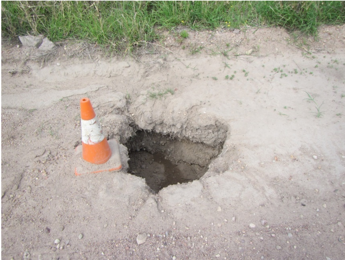
Figure 3-5. Tunnelling over LW12/15 on track adjacent NWCD associated with subsidence crack
