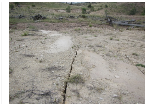
Compression buckle cracks at 1-2m spacing through the sandstone in NWCD near Div8 over LW 13/14 (2018)
