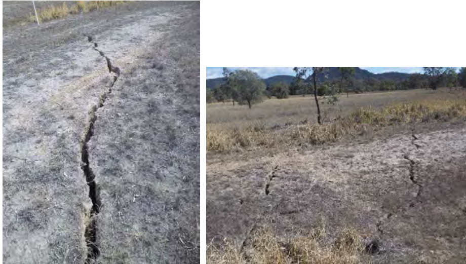
Fig. 4.7 Surface cracking above the middle of WYLW17
