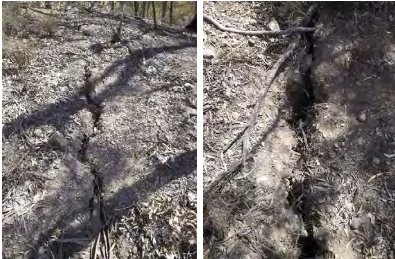
Fig. 4.8 Surface cracking on the steep slopes above the south-western end of WYLW17
