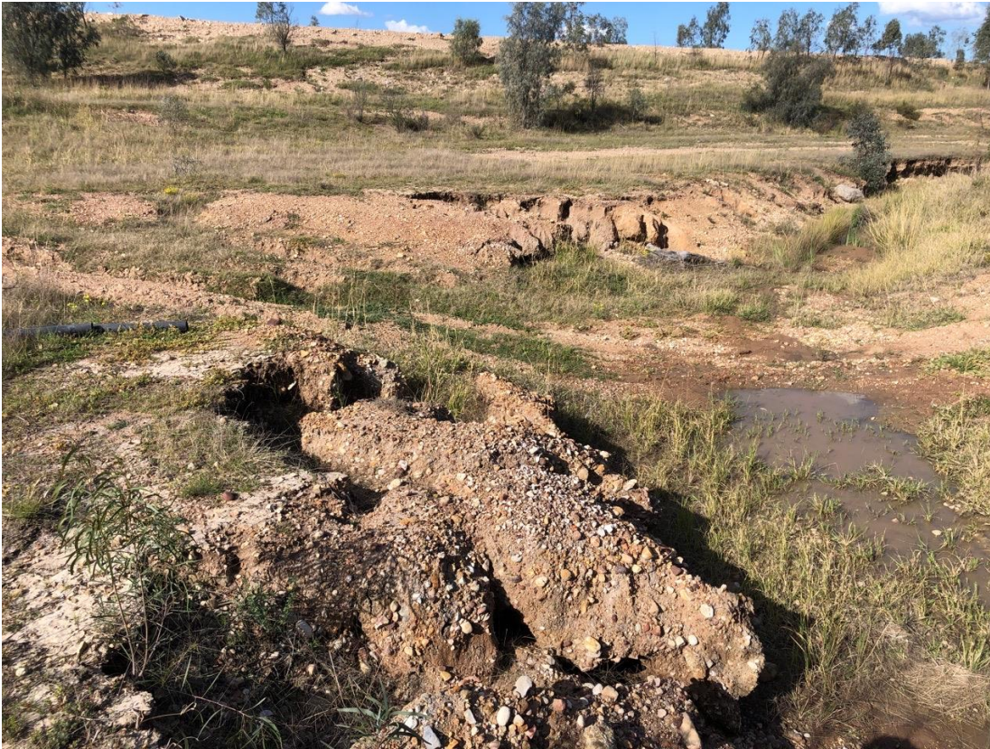
Photograph 43: Erosion issues along the North Wambo Creek Diversion near site 23R
