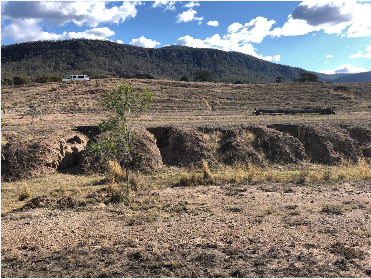
Plate 20: Gully erosion within the North Wambo Creek Diversion (near site 23R)
