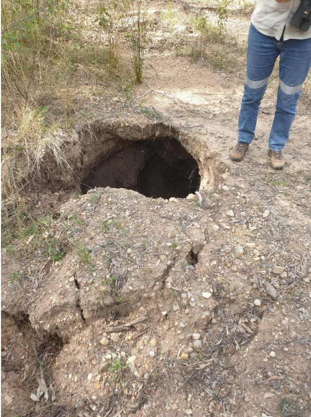
Photograph 34: Large hole on edge of track within RWEA C
