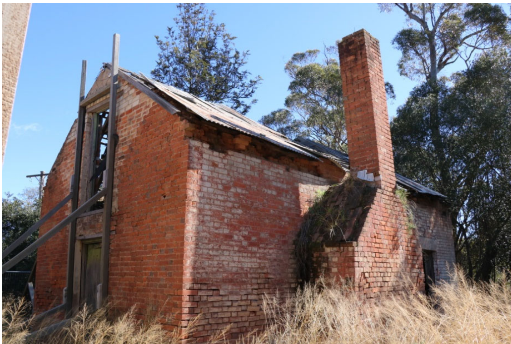
Figure: Advanced erosion of joints and loss of roofs 2017
