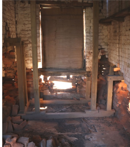
Figure: Collapsed brickwork and timber propping, north west corner. Source: EJE 2017
