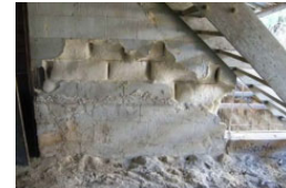
Salt damp attacked stonework
