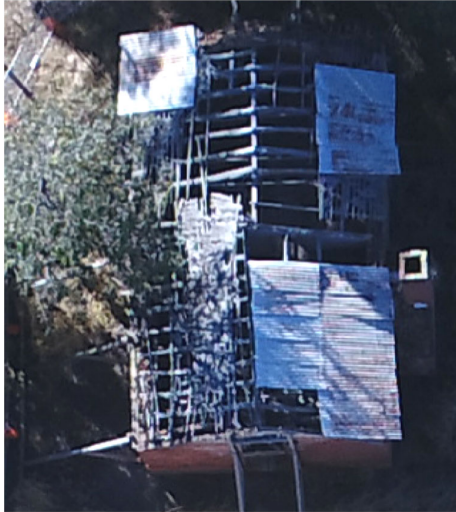
Figure: Servants' Wing Roof remnants. Source: Peabody Energy 2017
