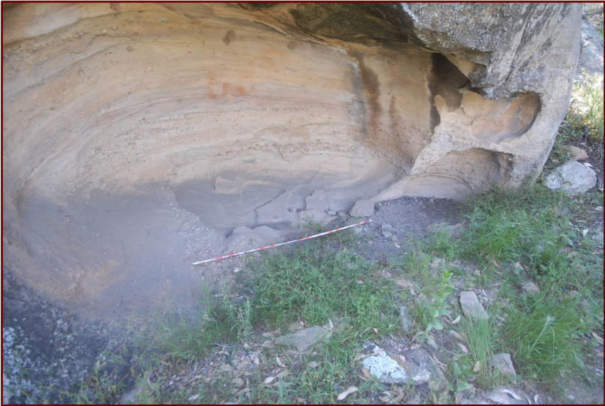
Figure 21 General view of the WCP153 floor, growth of herbs and grasses, and previously noted loose tabular surface rock, sourced from adjacent side slopes (DSC_0353).
