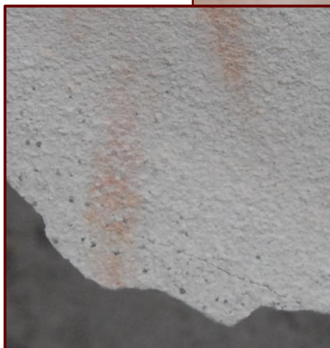
Figure 9 Detail of a newly noted hairline crack located immediately to the left of the recent detachment.
