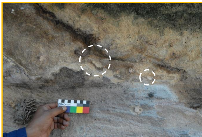
Areas of exfoliation noted in 2017 (DSC_0331)
