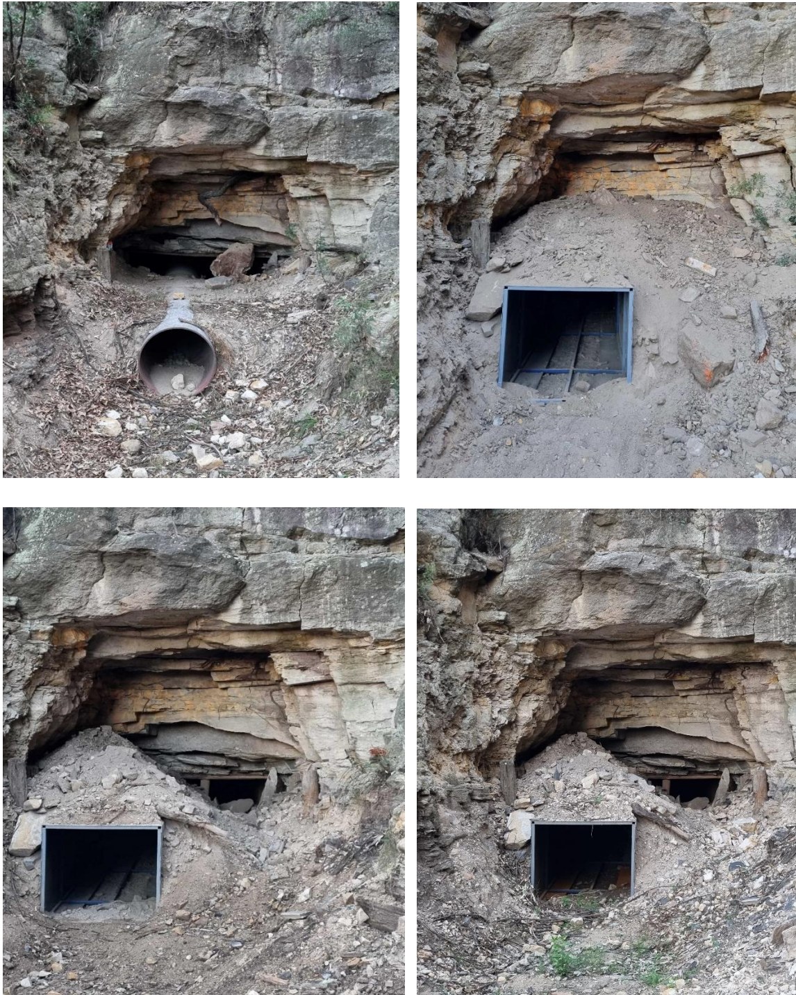
Plate 5-2: Monitoring photos of adit entrance pre culvert installation (March 2023 – top left), afternoon of installation (April 2023 – top right), three months after installation (July 2023 – bottom left), and nine months after installation (January 2024 – bottom right). This shows progression of pipe to tunnel with small aperture, tunnel with large aperture.
