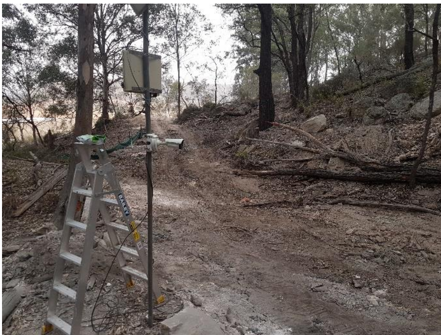
Plate 2-1: Slate Gully adit entrance prior to installation of steel pipe to maintain opening in the event of a collapse (mid 2019), also prior to installation of steel box tunnel (Apr 2023). Detector and solar panel setup 20m in front of adit.
