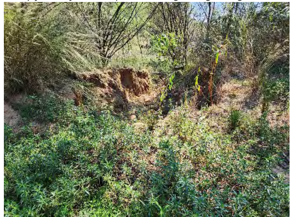
The embankment of the farm dam has already breached and may be subject to rapid failure in future flows.
