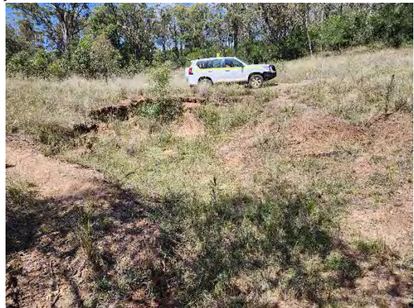
Existing erosion of valley fill where tributary crosses LW24-25 pillar. Further erosion in response to subsidence likely.
