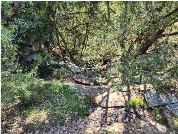
Bedrock cascade on tributary above farm dam where it crosses out of LW24 would limit any potential adjustment should the dam embankment erode further
