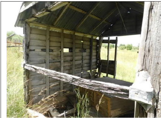
Figure 26: South facade of small shed where virtually all of the cladding has detached. The centre rail appears to be at a sill height and metal flashing around the ends of the rail seem to confirm this. The wall head however shows evidence of former wall studs.
