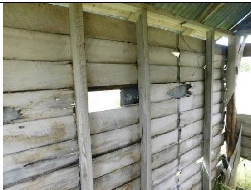
Figure 30: Weatherboards have suffered damage and have been patched. Termite damage to the post in the northwest corner is clearly obvious as the outer layer of the post is peeling away.
