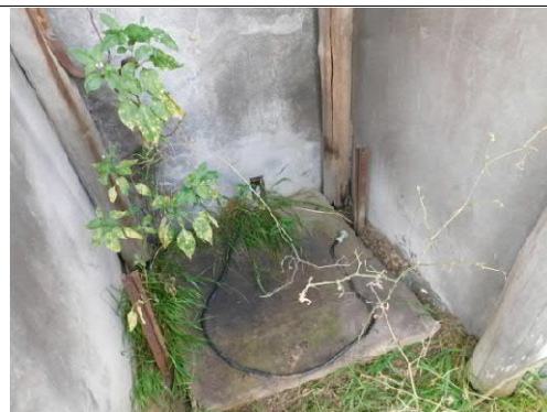
Figure 35: The floor of the pump shed with the power cable. There is no hole or plumbing connection.
