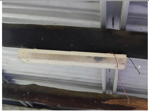
Figure 19: Fluorescent light fitting in the centre of the space shows occupation during the last 40 years. Note also the roof battens of folded metal and the Zincalume roof sheeting.
