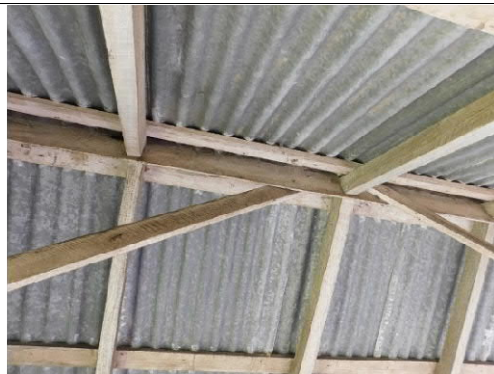
Figure 29: The roof structure of the small shed does not make allowance to hang objects such as carcasses for butchering from the ridge member.
