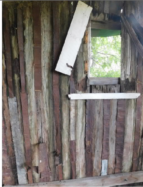
Figure 17: Looking up into the Hayshed roof showing the bush pole rafters and bracing.
