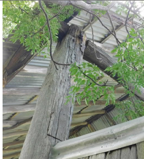
Figure 13: Hayshed post showing weather damage at the junction of the roof beam.
