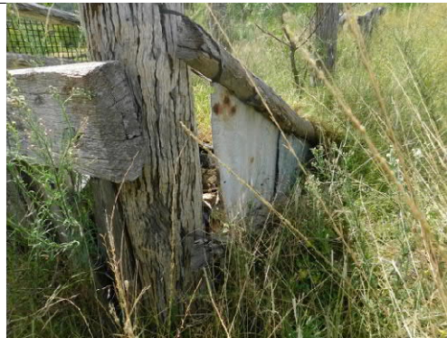
Figure 41: a detail of the loading ramp section of the Yards. Note the condition of the posts.
