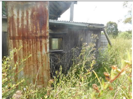
Figure 23: East facade northern half showing the door from the outside and the water tank beyond.
