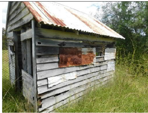
Figure 27: West facade of small shed showing weatherboards repaired with sheet metal. Barge roll of roof edge is visible at top left.
