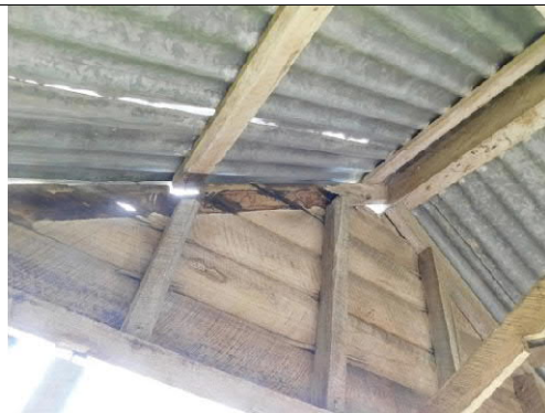
Figure 31: The northern gable of the small shed. The termite damage from the NW post continues into the gable structure where the member has been eaten out and collapsed.
