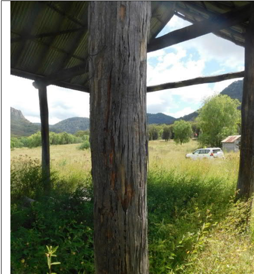
Figure 12: Hayshed post showing serious termite damage.
