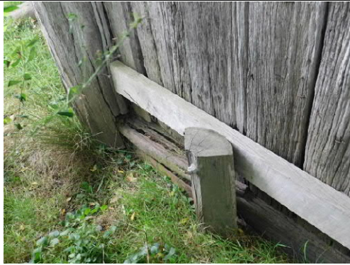
Figure 20: The southern wall has been repaired with treated timber rails inside and out with galvanised bolts through treated timber pegs driven into the ground
