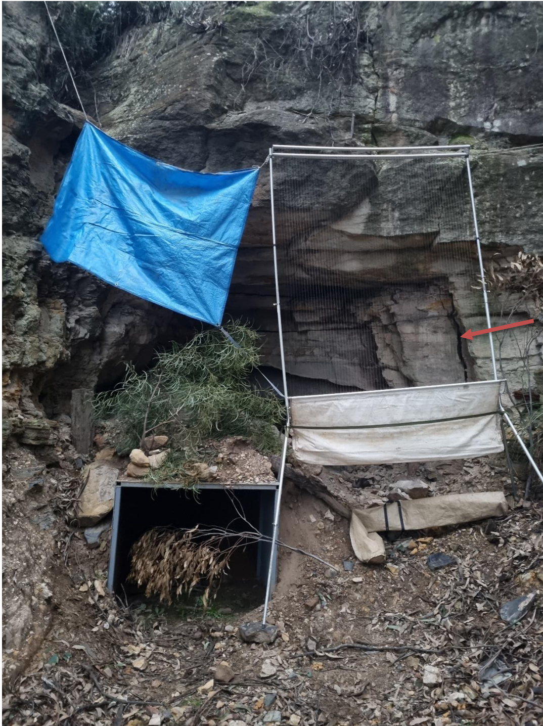
Plate 5-C: Monitoring photos of adit entrance 15 months after installation (July 2024). Harp trapping was conducted to get an update on roost status (species present, sex ratios and recapture of banded individuals). Large crack forming on western side shown with red arrow.
