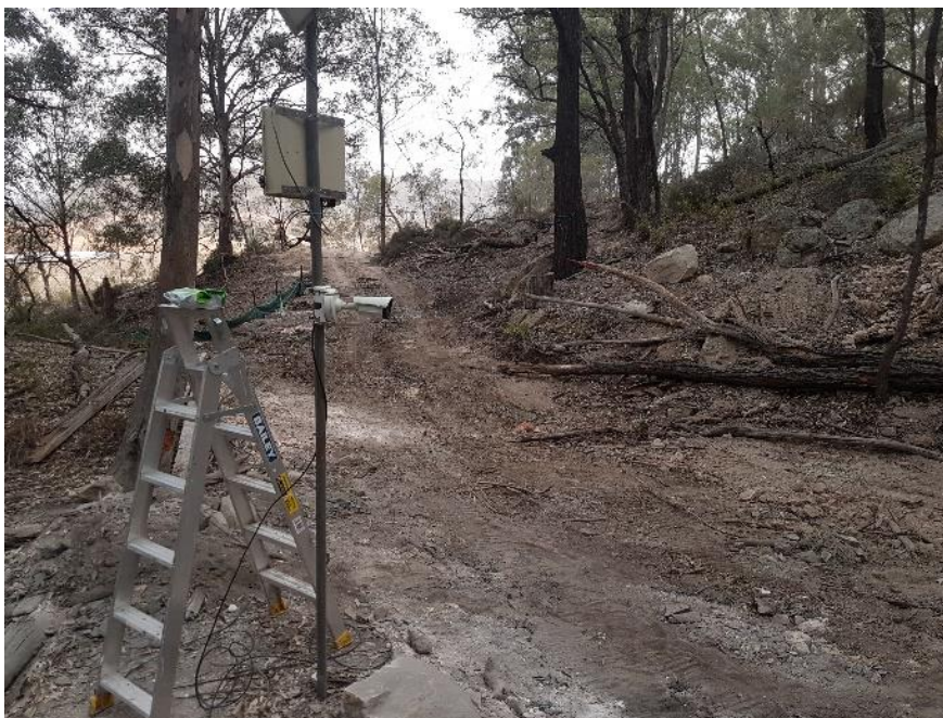
Plate 2-A: Slate Gully adit entrance prior to installation of steel pipe to maintain opening in the event of a collapse (mid 2019), also prior to installation of steel box tunnel (Apr 2023). Detector and solar panel setup 20m in front of adit.
