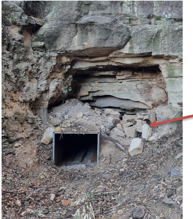
Plate 5-D: Monitoring photo of adit entrance almost three years after installation (April 2025). Shows rock collapse in bottom right (western side – red arrow).
